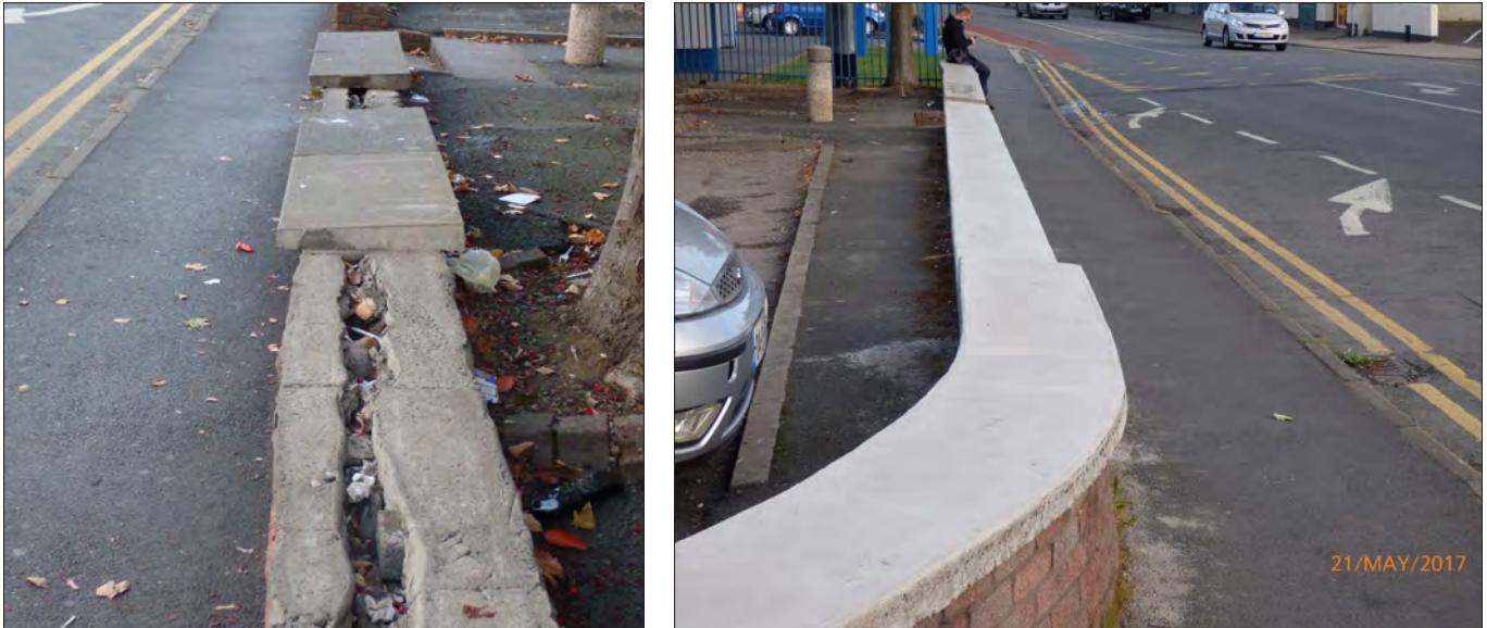
AXA INSURANCE - DUBLIN ROAD (NORTHERN ENTRANCE TO BRAY) BEFORE AND AFTER RE-CAPPING OF WALL.
